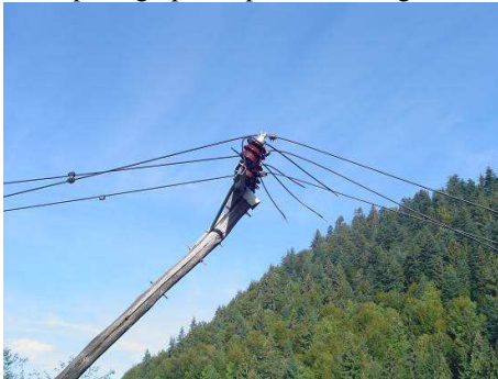
Figure 1: Suspension pole with ceramic insulators.
