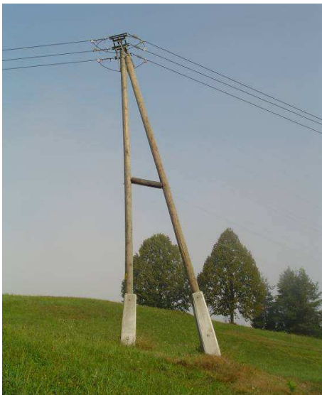
Figure 2: Pulled out tension pole.
