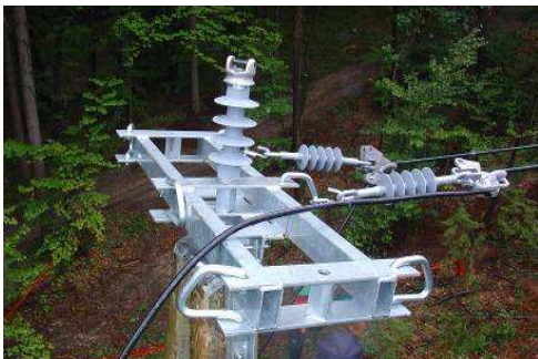
Figure 14: Undamaged tension pole.
