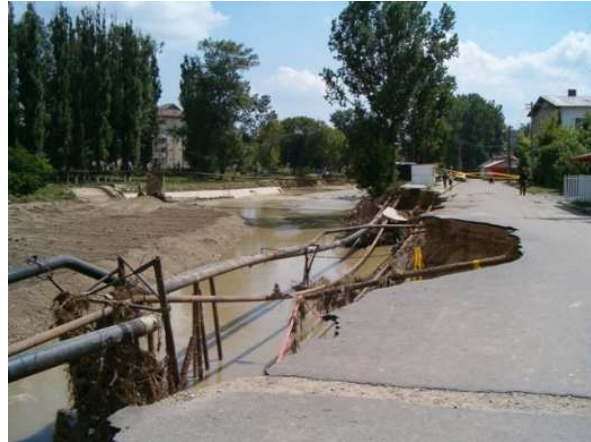
Figure 6. Bank erosion with MV affected cables
