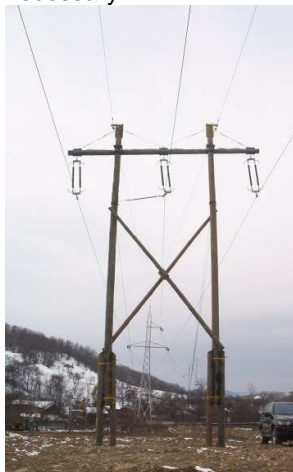
Figure 9. 110 kV portal wooden pillar
