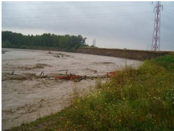
Fig. 4. 110 kV broken pillar fallen in Prahova river. The bank erosion caused by the abnormal water flow is visible
